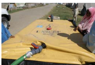
Water bladder installed by UNICEF at Sheikh Yaseen Camp
